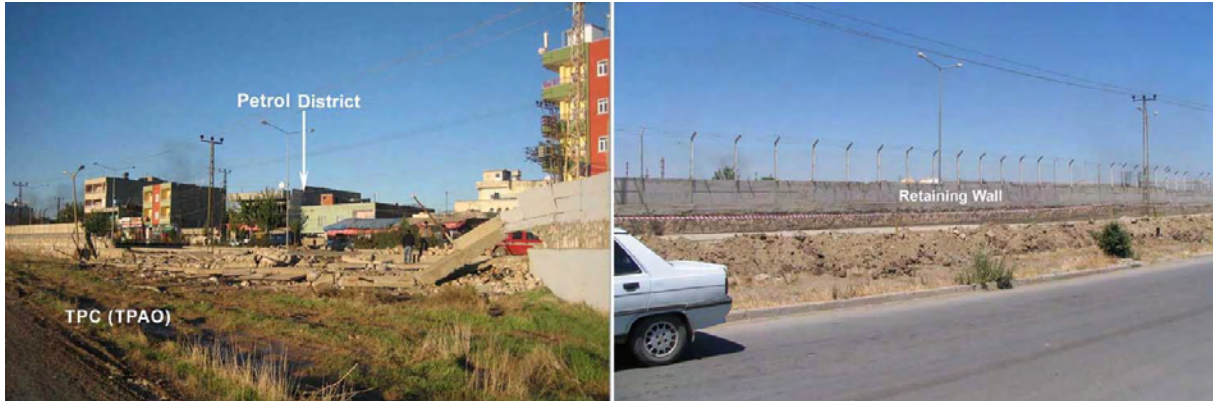
Figure 14. Retaining wall of Turkish Petroleum Corporation facilities demolished in the flood event on October 31-November 1 2006 and later rebuilt.
