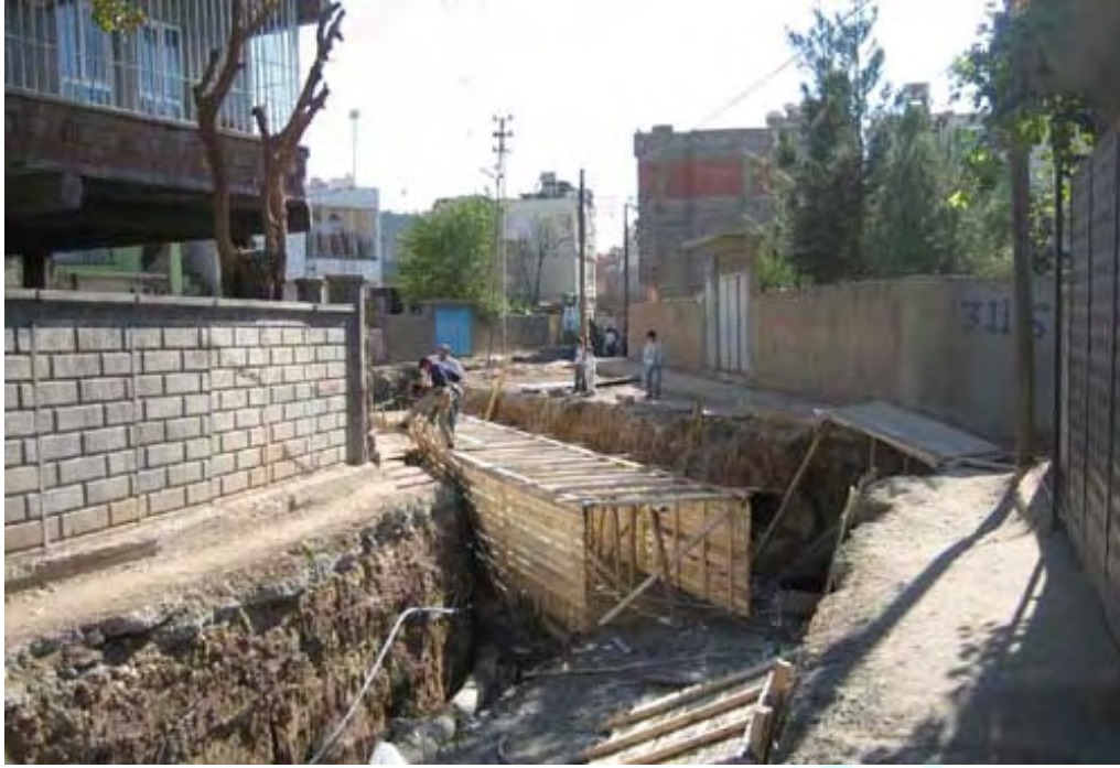
Figure 11. Dwellings constructed on a stream bed in the district of Karşıyaka and flood prevention works carried out in Street 311 after 2006.
